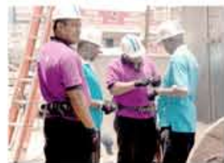
Photo 1: Employees from TSTT examine fiber optic cable in preparation for splicing and termination. Photo 2: During an exercise, workers prepare the fiber optic cable for termination.
